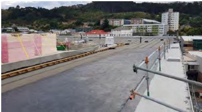
Roof vapour barrier complete to West and PIR & Poly stored on site
